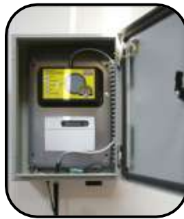
Sea Marshall Base Unit and auto dialer installed in a enclosure
